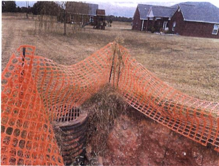
Pipe failure location looking towards 132 Bermuda Ln
