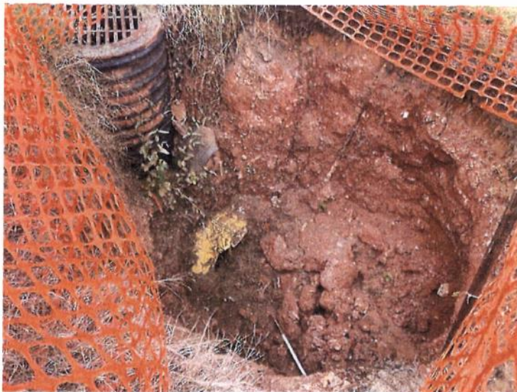
View inside hole caused by pipe failure
